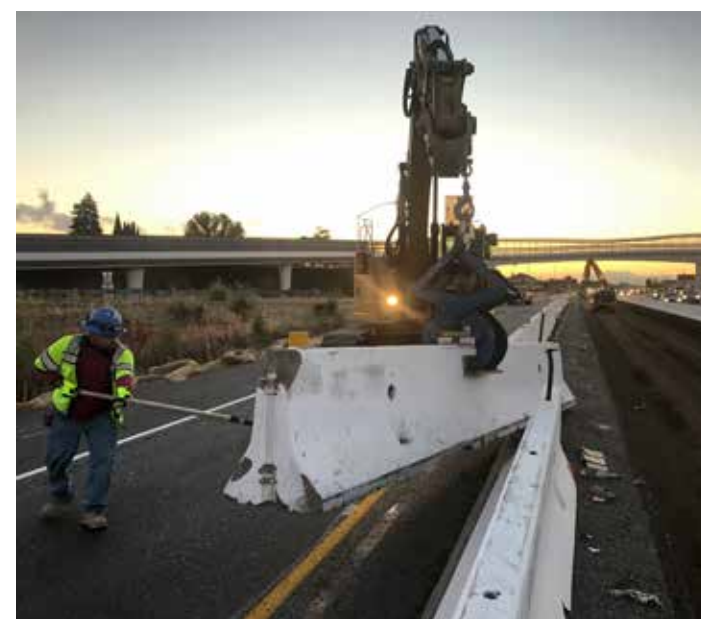
K-rail was set in place as protective barriers against the traffic that surrounded crews on site.
