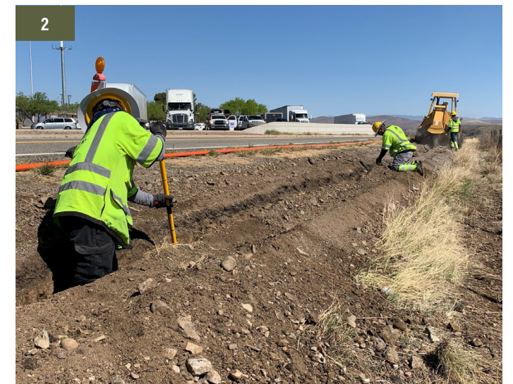
1. Conduit was installed on steep, mountainous terrain through off-road trenching alignment 2. Crews use a rock saw trencher and actively check the depth of the trench prior to placing the conduit.
