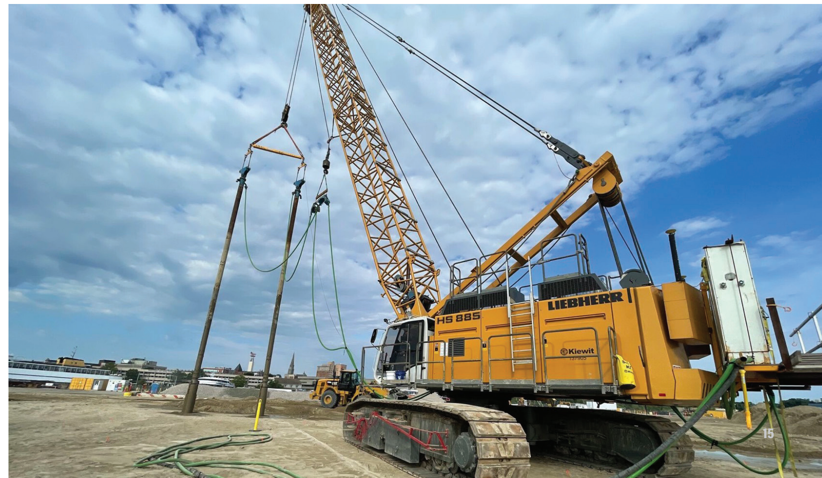
Vibro-compaction was completed with a dual-probe set-up on the Connecticut State Pier project.
