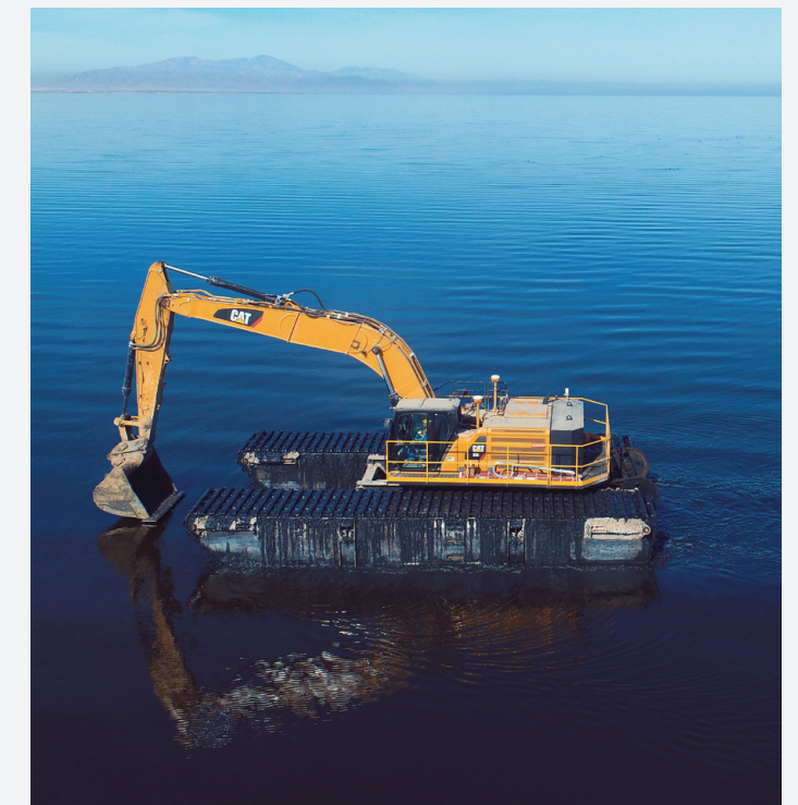
Here is a pontoon excavator, a key piece of equipment on the project. It's amphibious and able to go to the most difficult areas of the project.
