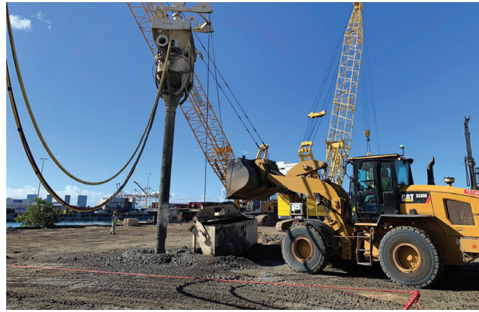
Crews at Kapalama self-performed the stone column work. The incorporation of stone columns to reinforce soils against seismic loads and liquefaction is relatively new for Hawaii Department of Transportation designs.
