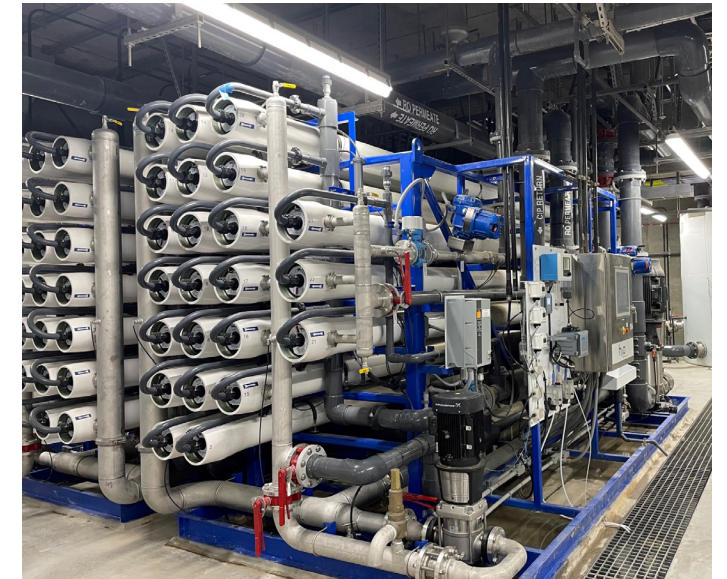
The Advanced Water Treatment Facility can treat up to 1.2 million gallons of wastewater per day.
