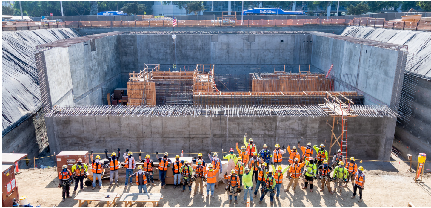
Kiewit's workforce on the project peaked at 13 staff and nearly 70 trade craft employees. Subcontractors brought the total craft workforce to nearly 100.
